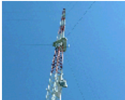
Lansing Civil Defense Repeater Association
